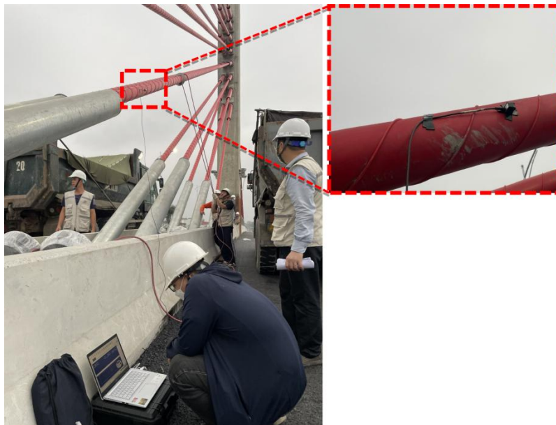
Fig. 13 – Arrangement of cable vibration measuring equipment
